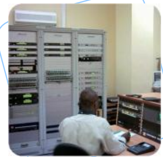
Exploitation room of a DVB platform
